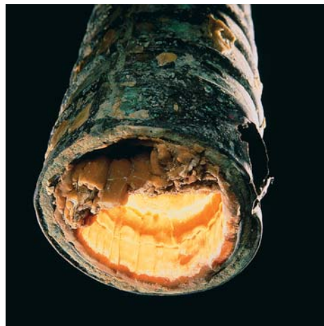
Boiler scale almost fills this hot-water pipe. The deposits consist mostly of \text{CaCO}_3 with some \text{MgCO}_3 .
