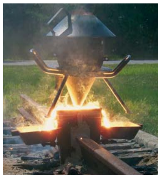
The molten iron formed in a thermite reaction is run down into a mold between the ends of two railroad rails. On cooling, the rails are welded together.
